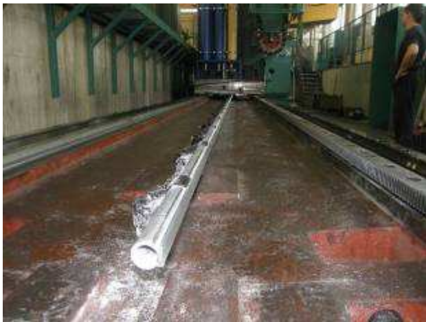
Photo showing use of composite thermally stable measuring on the WRD150 duo machine, combined with a concrete base for the machine through openings in the machine bed
